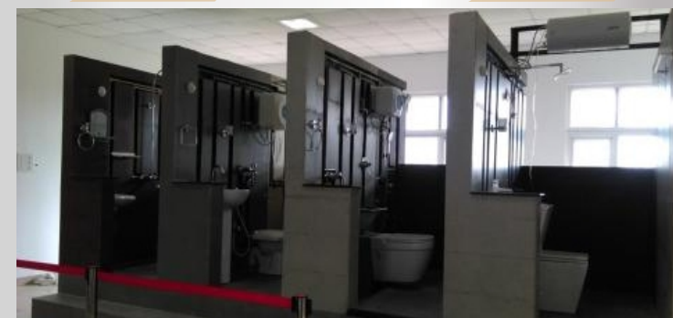
Plumbing Training Centre at Don Bosco, Bangalore
