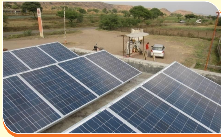
IOC's Solarized KSK: M/s Kakad Brothers, Thanegaon, Maharashtra
