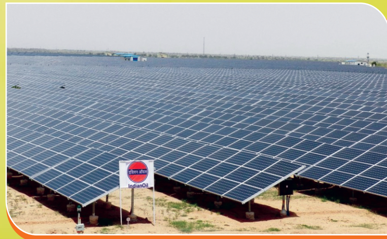
IOC's 5-MW solar power plant at Rawra, Rajasthan
