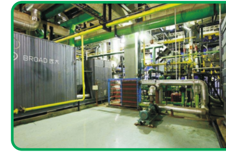
Gas Co-generation System
