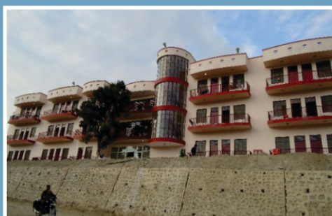
Construction of girl's hostel for students studying in THDC-Institute of Hydro Power Engineering & Technology at Tehri, Uttarakhand
