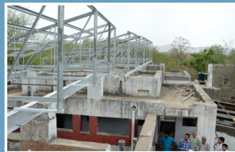
Installation of 135 KWP off-grid solar plant in campus of the SWRC (formerly known as Barefoot College), Tiloniya" in Ajmer district of Rajasthan.
