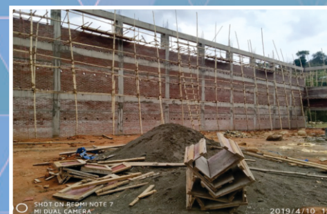
Construction of multipurpose hall cum indoor stadium in Somdal village in Ukhrul district, Manipur
